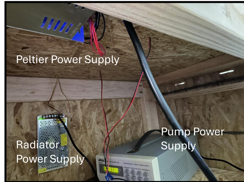
Figure 18: Power Supply Setup
